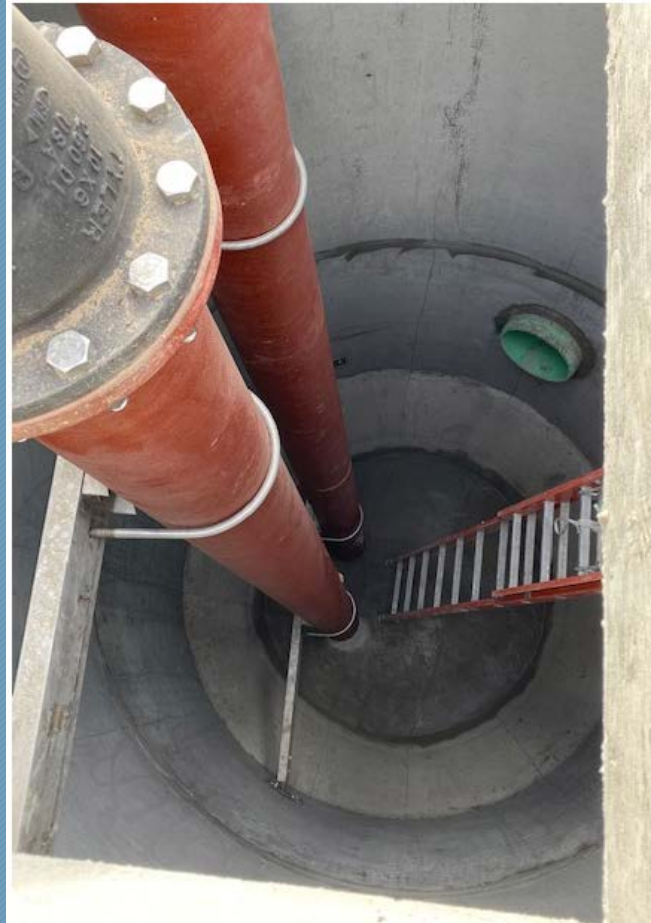
Suction Pipes from Wet Well
