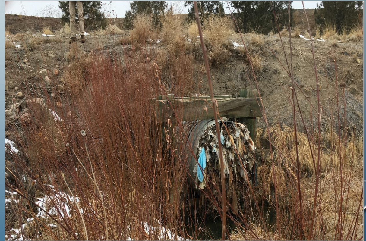
Clogged Storm Drain Downstream of Landfill
