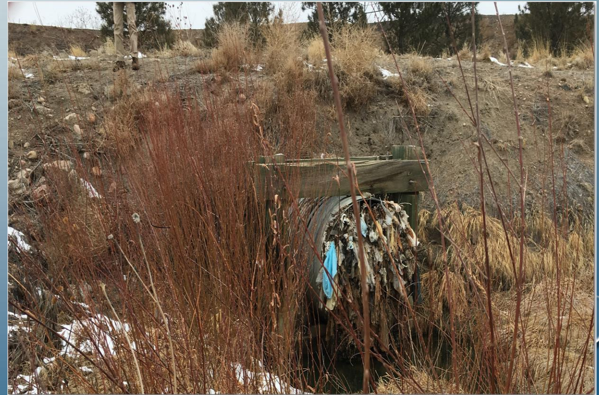
Clogged Storm Drain Downstream of Landfill
