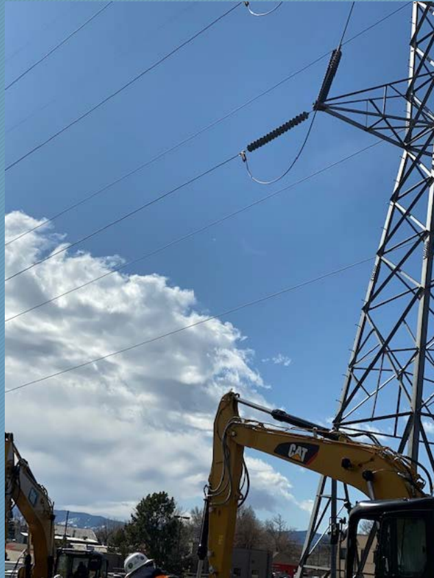
Working Near Power Line
