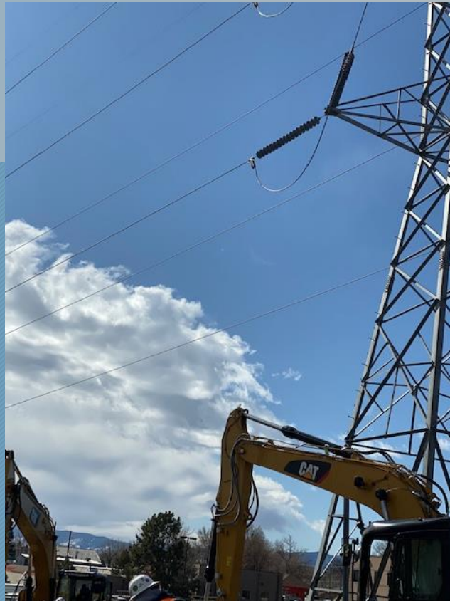
Working Near Power Line
