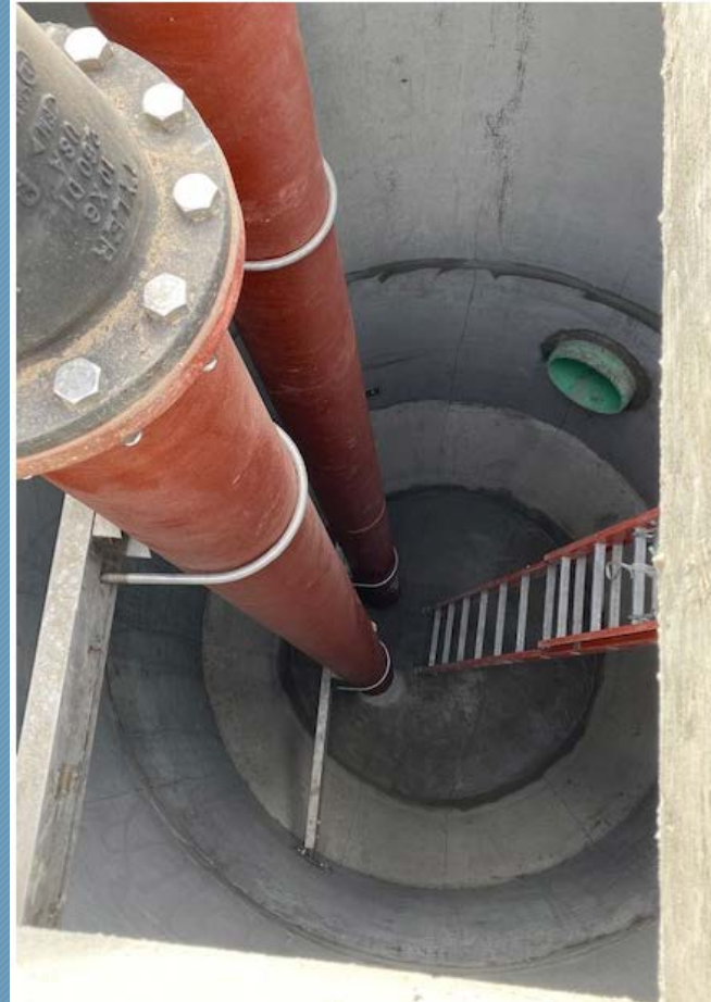
Suction Pipes from Wet Well
