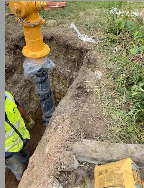
Hydrant on Canyon Dr
