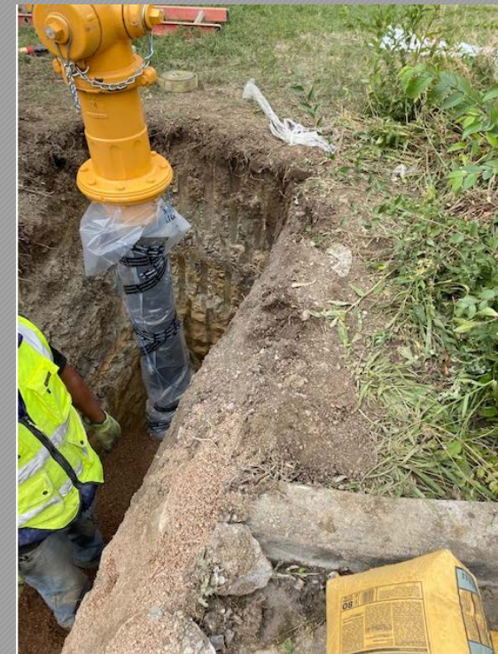
Hydrant on Canyon Dr
