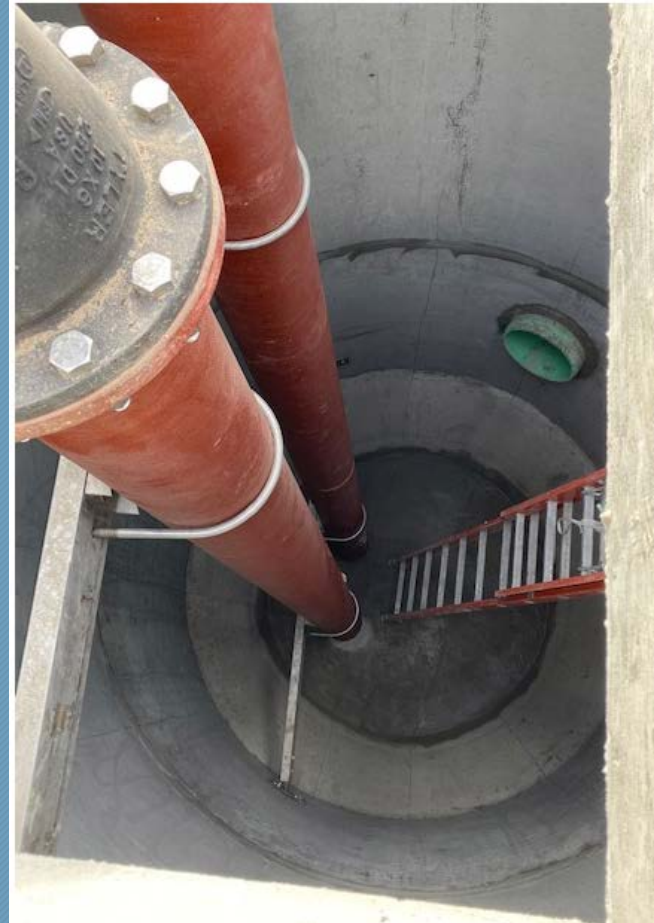
Suction Pipes from Wet Well
