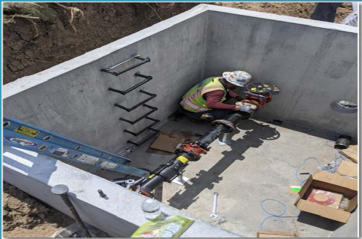
Irrigation Service Through Vault
