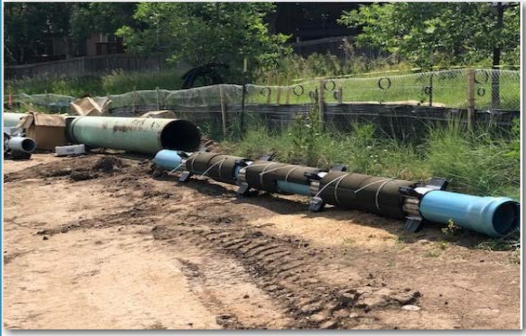
8" Sewer Main with Insulation and Skids
