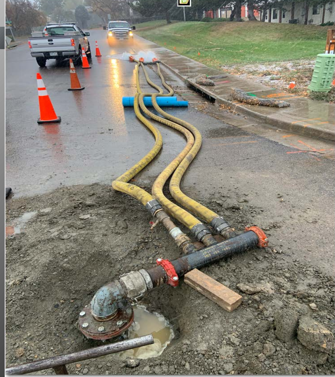
Flushing manifold after 4 failed tests
